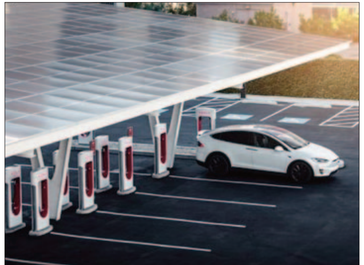
The installation of electric vehicle charging stations is a point of discussion for the OVTD Energy Solutions Committee.
