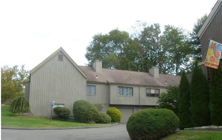
Photograph 3 Note staining on roof shingles.
