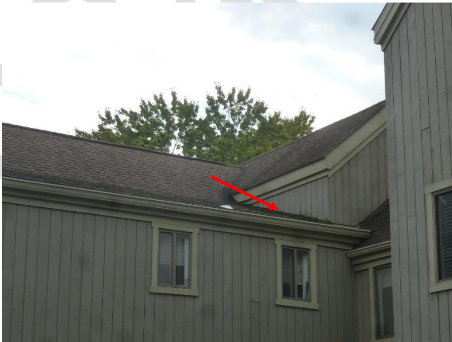
Photograph 12 Note inadequate clearance between roof and siding.
