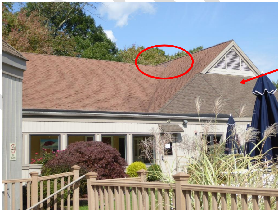
Photograph 2 East Side Roof – North Clubhouse (Note new/old shingle intersection above lower ridge and newer roof section replacement)
