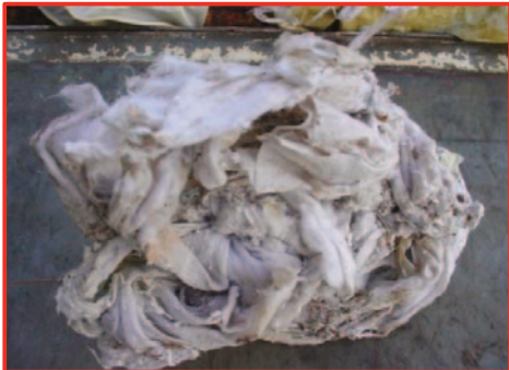
Mounds of wipes removed from a clogged pump at the Willow Brook Pump Station, New Britain.
